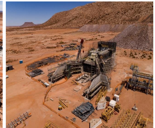
ROM - Primary Crushing
